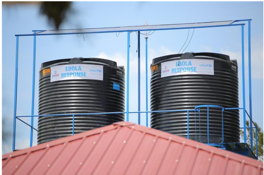
Figure 3: Installed water tanks in Mubende to supply water to treatment and isolation centres. Credit: © UNICEF/2022/Joseph Balikuddembe
